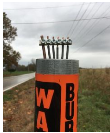
Floating Ground Buss.
